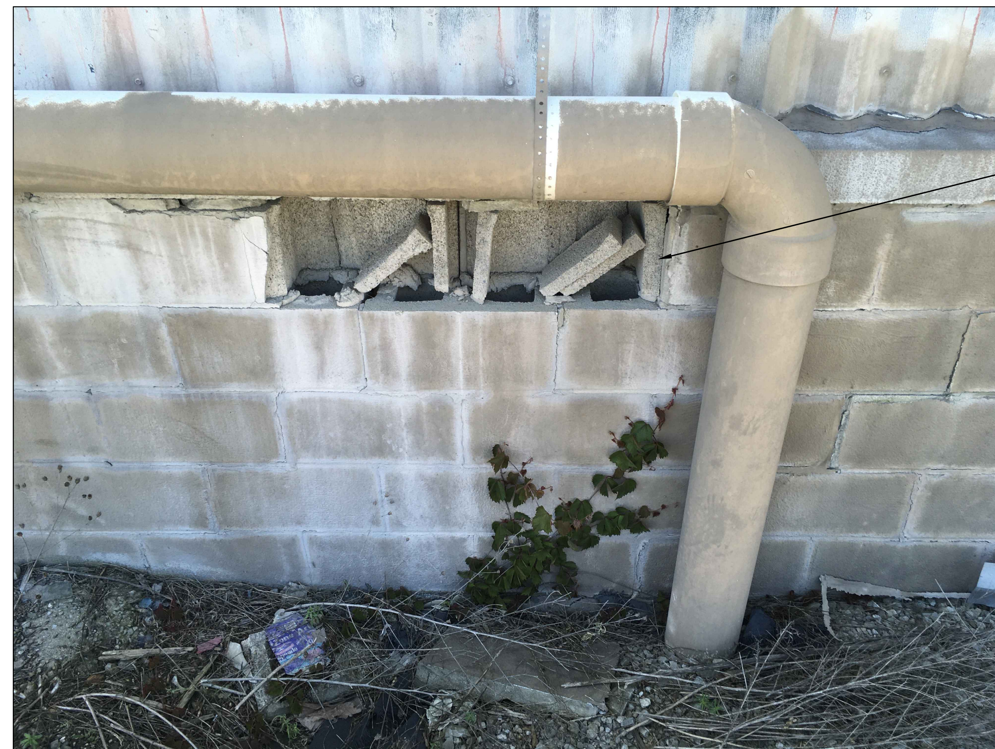
3 TYPICAL BROKEN CMU BLOCK R-101 NOT TO SCALE
