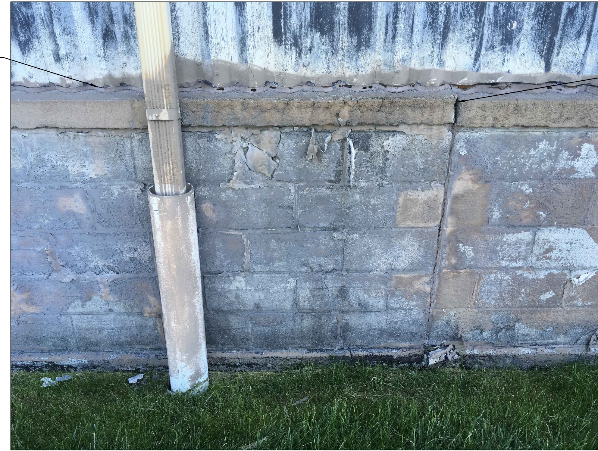
2 TYPICAL DETERIORATED SEALANT R-101 NOT TO SCALE
